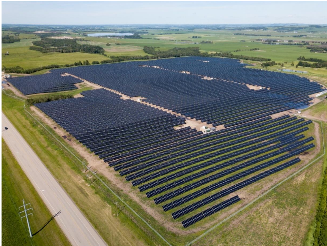
Elemental Energy Inc. Innisfail Solar FarmSOLAR.
