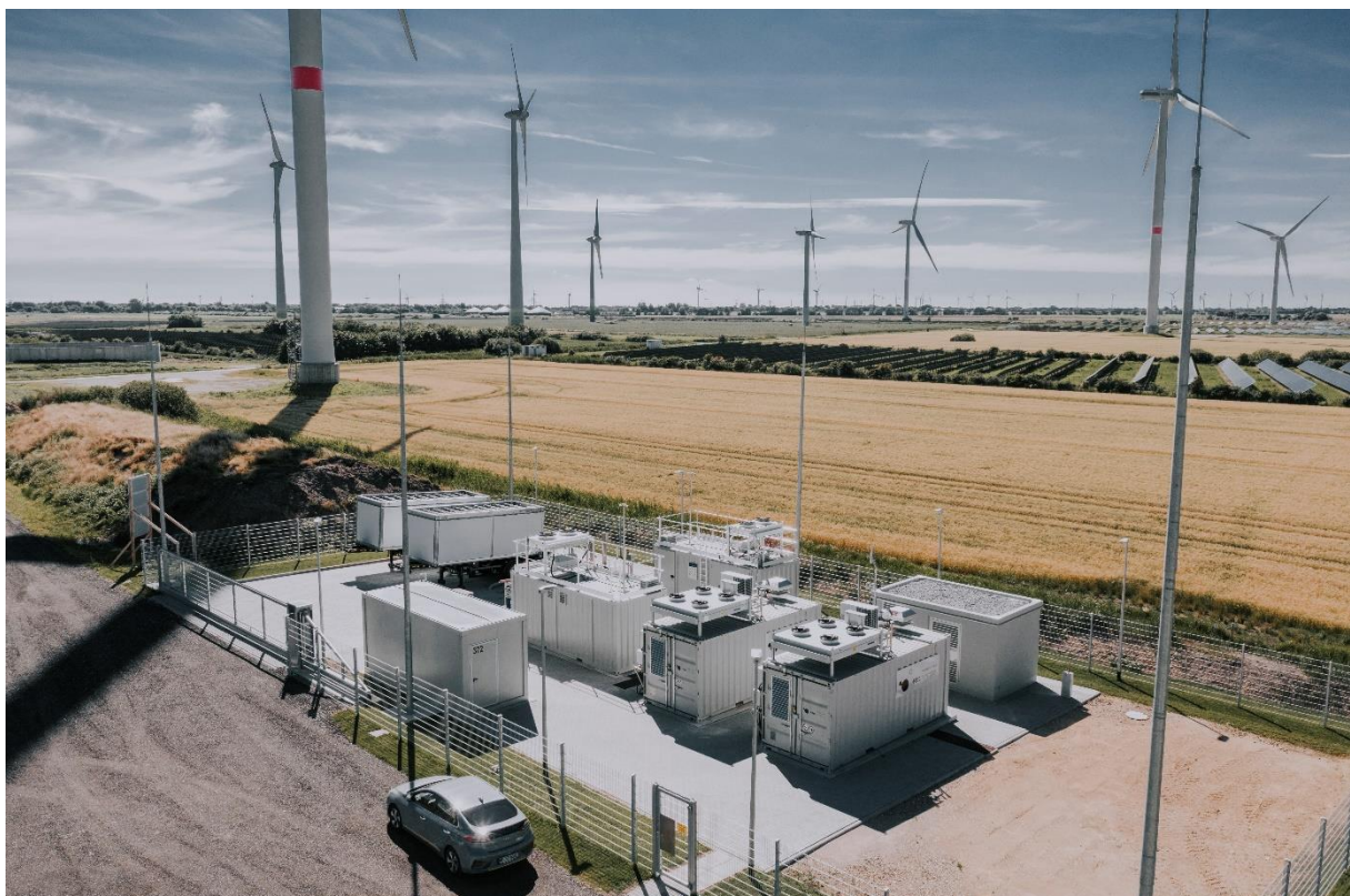
BU2 Bosbüll in North Frisia: Wind power and electrolysis in one location.
