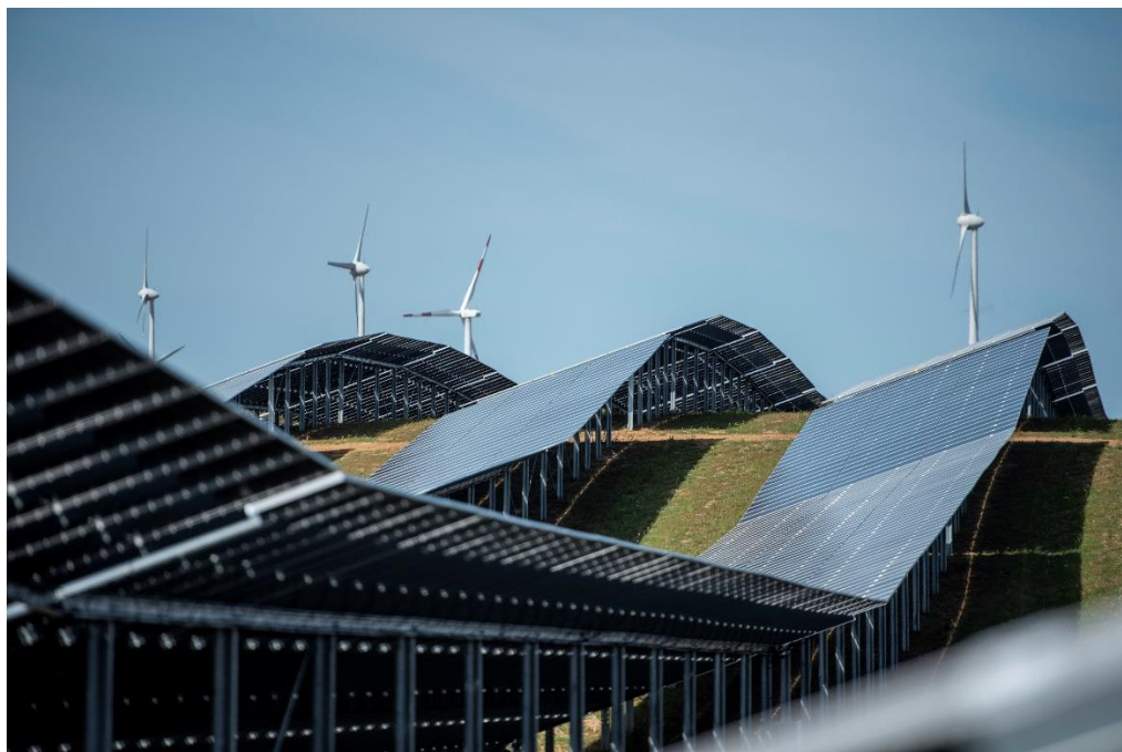
Caption 3: Special precision was required during assembly to take the terrain into account.
